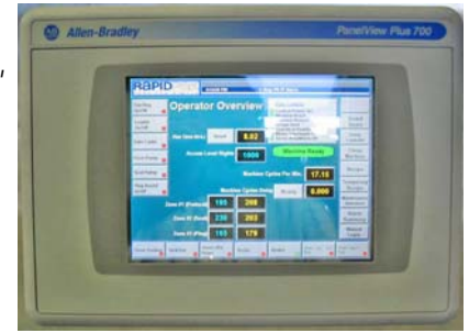
Allen Bradley Parallel Plus Touchscreen
